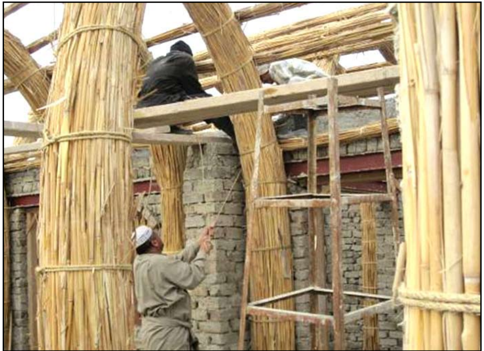
Iraqi contractors construct the main reed arches of a marsh Arab mudhif. The house is a blend of adobe and reed building materials used frequently by marsh Arabs in southeast Iraq. U.S. Army photo courtesy of the 4th Brigade Combat Team, 1st Armored Division.
